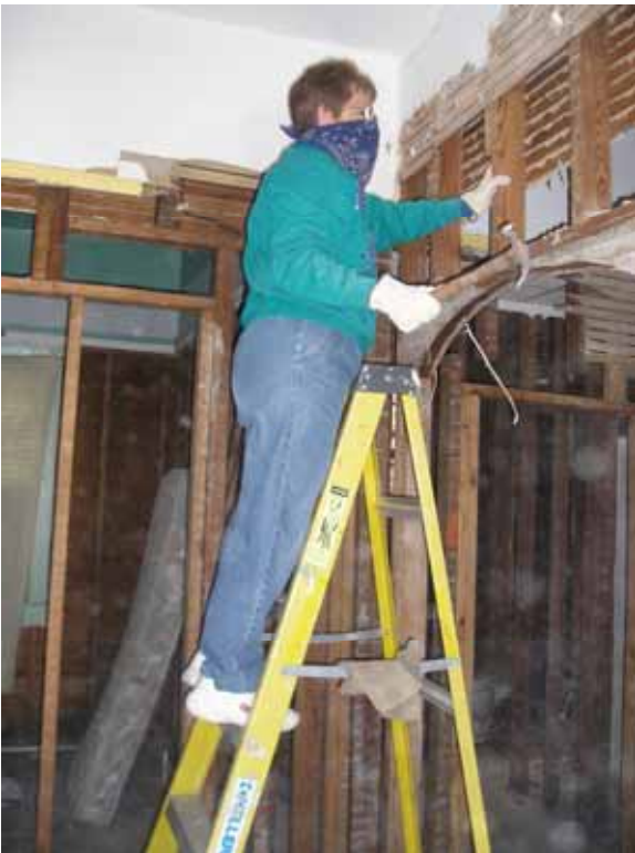
Garmane Mack's house: Sister Maureen gets into the swing of things by helping strip off damaged plaster.
