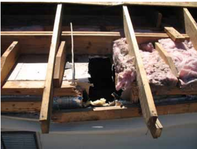
Damage to Lee's house
